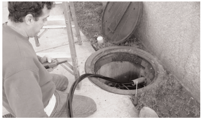
Electrician pulls new electric service wire for Boutwell House through underground conduit installed last December. Photo by Al Collins.
