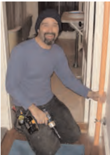
Mike and other pipe fitters from Fire Sprinkler Systems, Richmond, NH, have installed a full fire-suppression system throughout Boutwell House. Photo by Al Collins.
