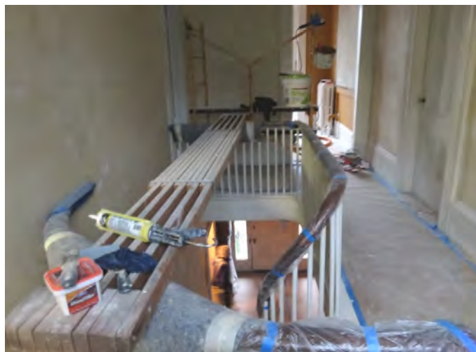
Stairwell and halls upstairs and down have been stripped of old wallpaper and carefully prepped for paint. Photo by Barbara Murray.
