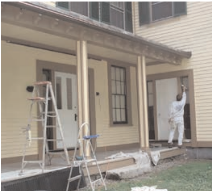
Side porch gets fresh paint prior to construction of a new ADA accessible walkway. Photo by Al Collins
