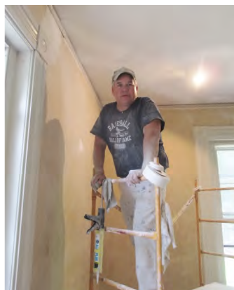
Dan Lowney preparing wall surfaces in the Grant bedroom to receive wallpaper. Photo by C. David Gordon
