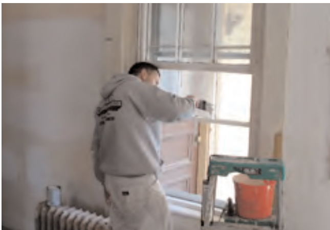
Boutwell House gleams with fresh paint, the work of Don Haberman and Son of Groton. Photo by Al Collins.
