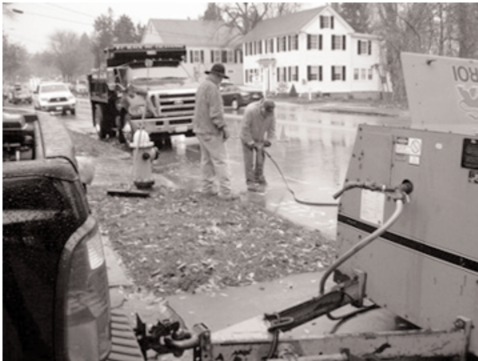
Installation of a water line for the new fire suppression system in Boutwell House began with jack hammering the street pavement. Photo by Al Collins.
