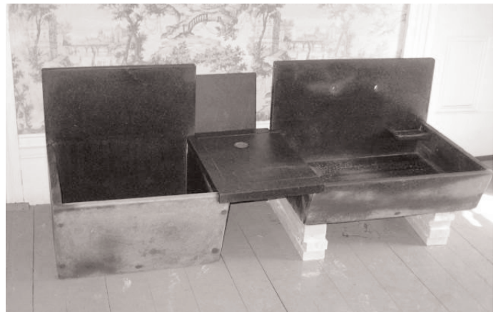
Restored soapstone sink awaits custom cabinet and period faucets before installation in Boutwell House kitchen. Photo by Al Collins.
